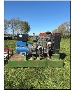
Marelli 3 Phase Generator - £1,750
